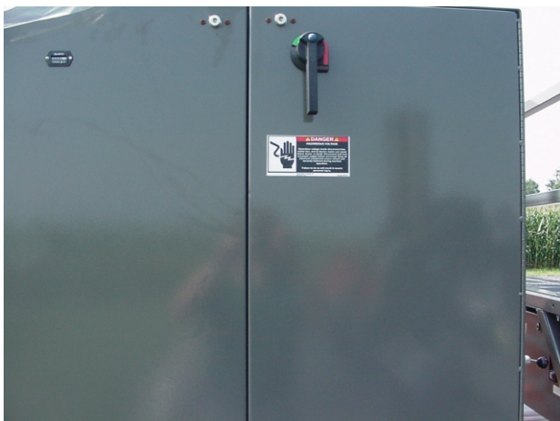
S20061 Decal, Electrical Hazard Danger
