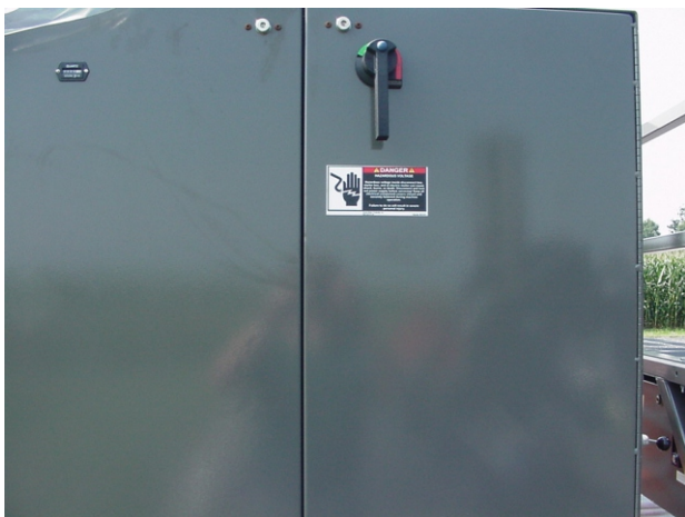
S20061 Decal, Electrical Hazard Danger
