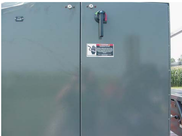
S20061 Decal, Electrical Hazard Danger
