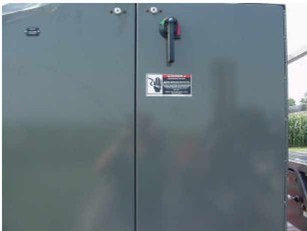
S20061 Decal, Electrical Hazard Danger
